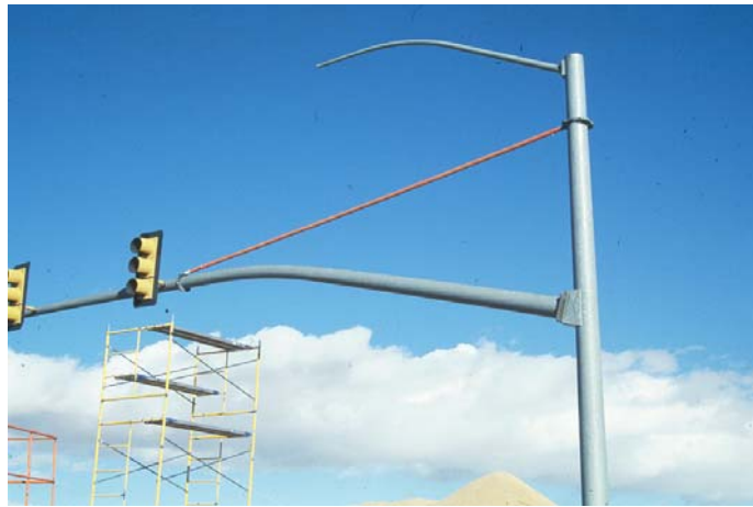
Figure 40. Wyoming Strand Damper.
