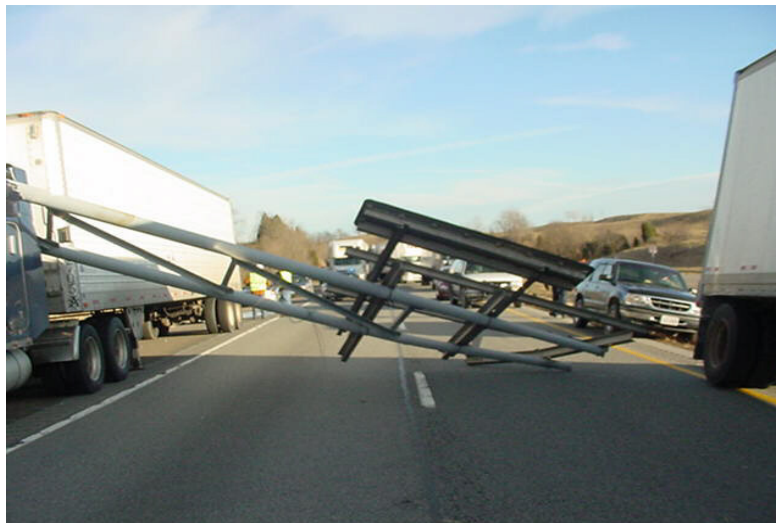
Figure 1. Cantilever Sign Structure Failure.
