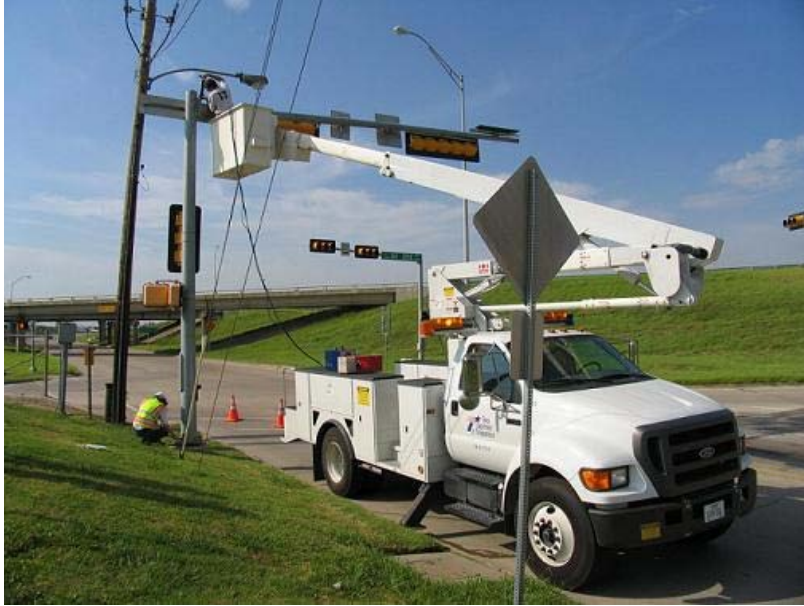
Figure 2.2 Mast Arm 1 on the Northeast Corner of the North Intersection of I-35E and Bonnie Brae Street in Denton, TX
