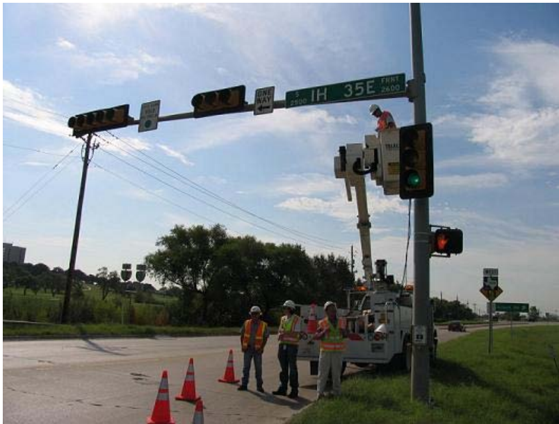
Figure 2.3 Mast Arm 2 at the Southwest Corner of the South Intersection of I-35E and Bonnie Brae Street in Denton, TX
