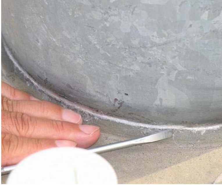
Figure 2.8 UIT Application at the bottom of Mast 2
