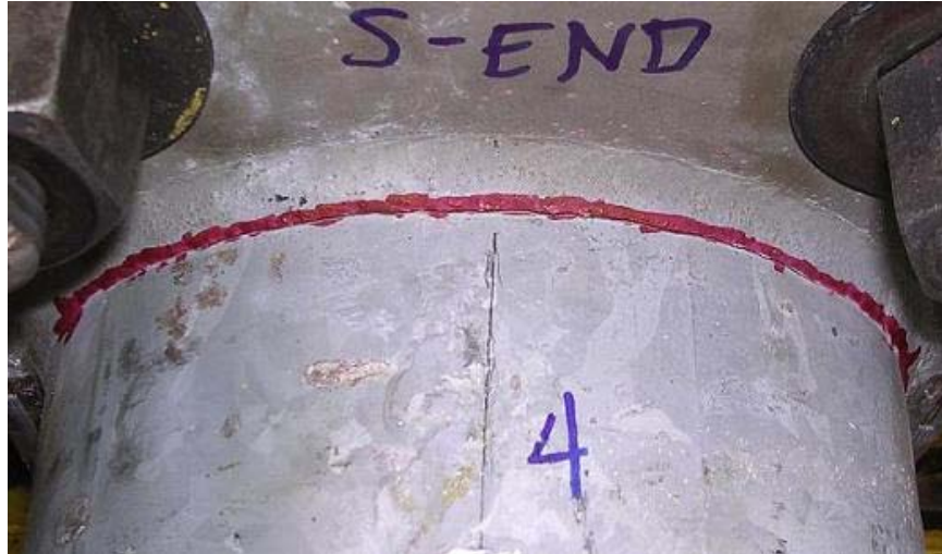
Figure 3.14 Highlighted Fatigue Crack Along Mast Arm Weld Toe of Specimen DN (224,905 cycles)
