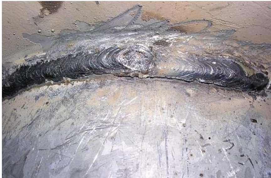
Figure 3.11 Close-up of Fatigue Crack on Specimen DU Mast Arm Weld Toe Along the Weld Repair (116,876 cycles)
