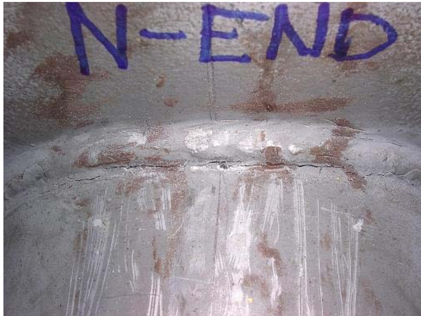
Figure 3.9 Close-up of Fatigue Crack on Specimen DU Mast Arm Weld Toe Along the UIT Application Line (90,680 cycles)
