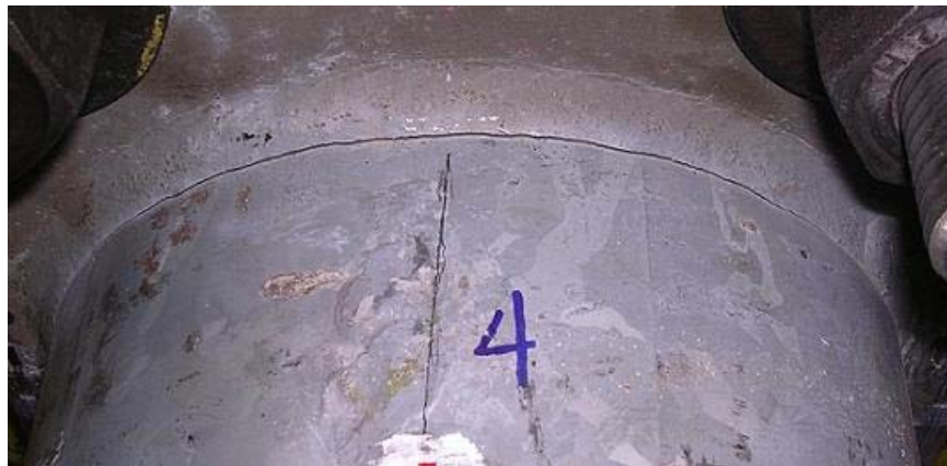
Figure 3.13 Close-up of Fatigue Crack Along Mast Arm Weld Toe of Specimen DN (224,905 cycles)
