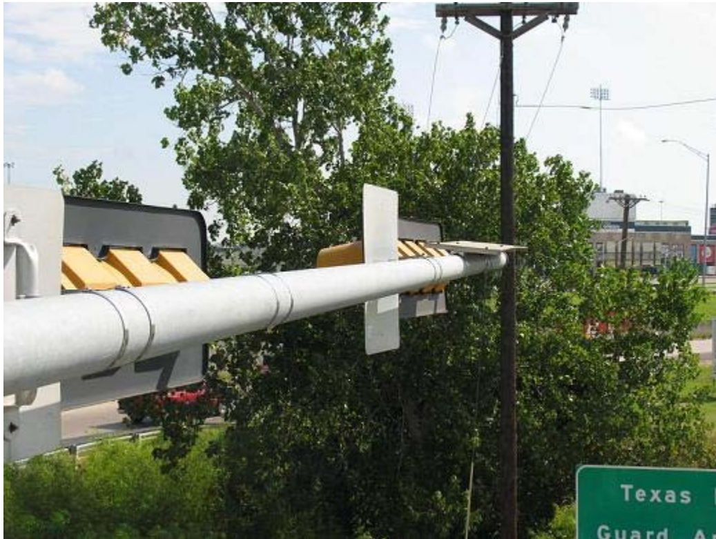
Figure 2.4 Horizontal Damping Plate on Mast Arm 2
