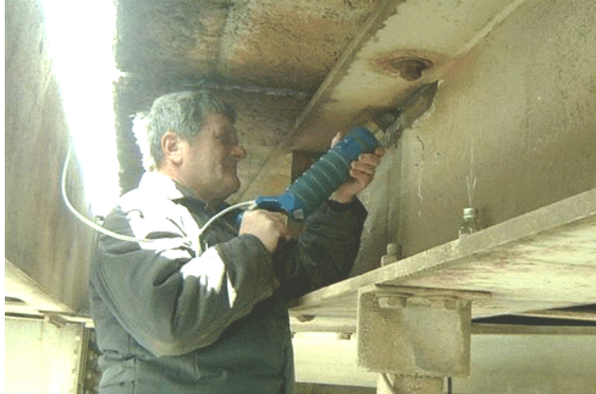
Figure 10. Photo showing the location of fatigue crack in welded element of bridge span and application of UP during the repair of crack
