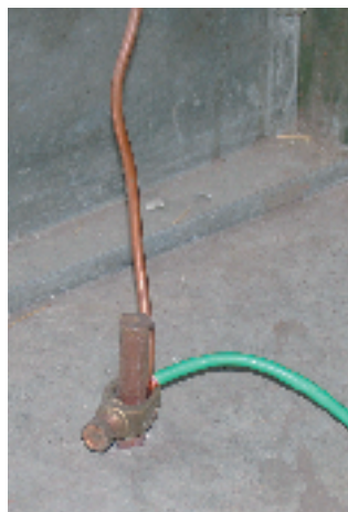
Ground to earth
