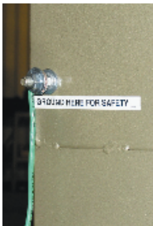
Ground from cabinet
