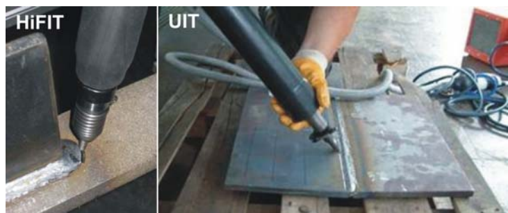
Figure 1: Application of air driven (HiFIT, left hand side) and ultrasonic excited (UIT) hammer peening processes (right hand side).
