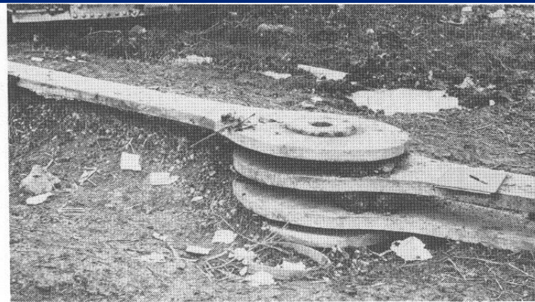
Figure 2.7 One of the eyebar joints after collapse (courtesy of Federal Highway Administration).
