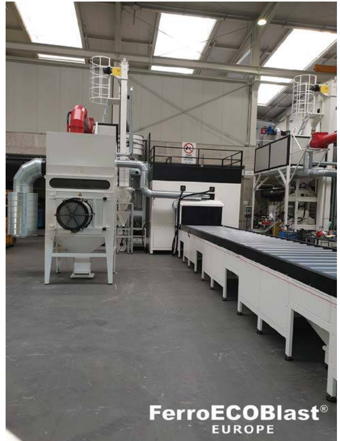
Conveyor for long parts and ATEX filter system
